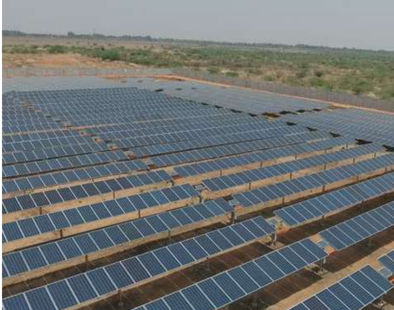
Fig3: Single axis solar panels tilt source: Mahindra sustain
