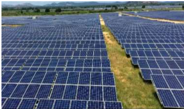
Fig2: Fixed solar panels that are placed with MPPT protocol
